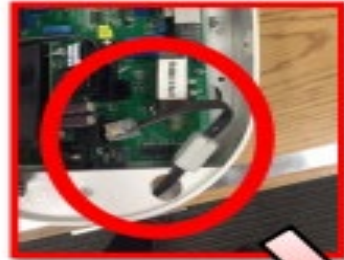
Power Board to Port: PB
